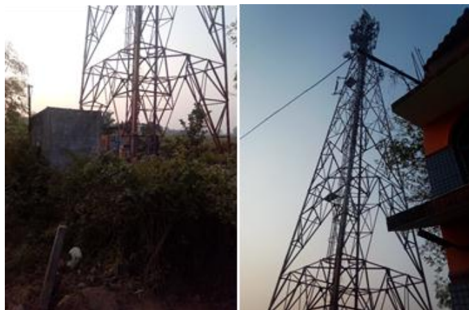
Figure-1: Cellular Base Transceiver Station (BTS)
