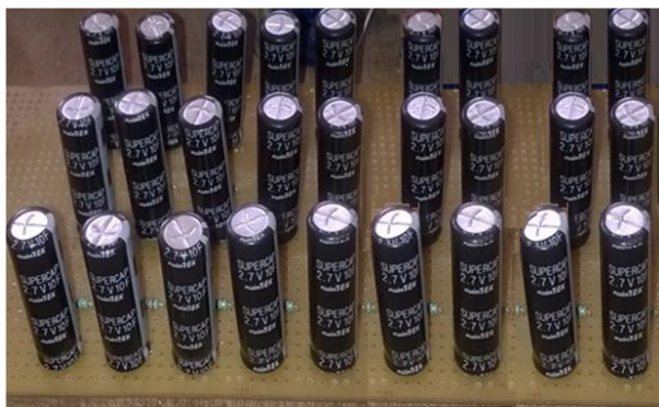
Figure.8. Ultra Capacitor Bank
