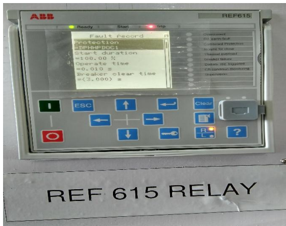
Figure 14. OC Fault Record
