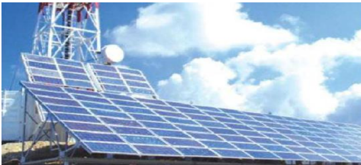
Fig 1: Photovoltaic cells (PV) at BTS Site [3].
