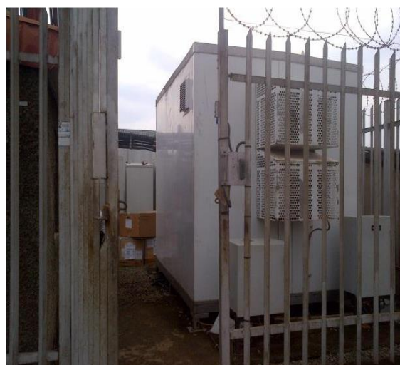
Fig 6: BTS Shelter for Indoor BTS
