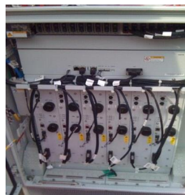
Fig 13: TRX's for 2G and 3G inside the BTS cabinet
