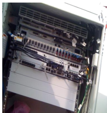
Fig 11: Top part of the inside of a BTS cabinet
