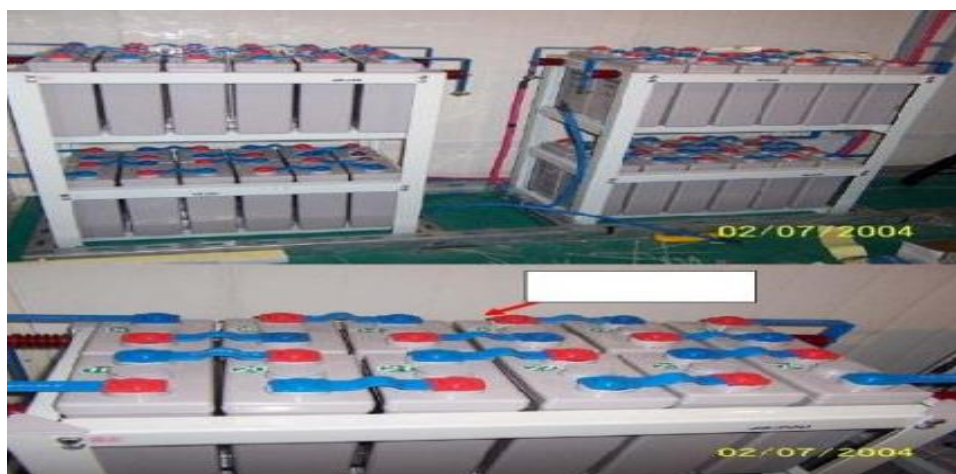
Fig 14: View of a Battery
